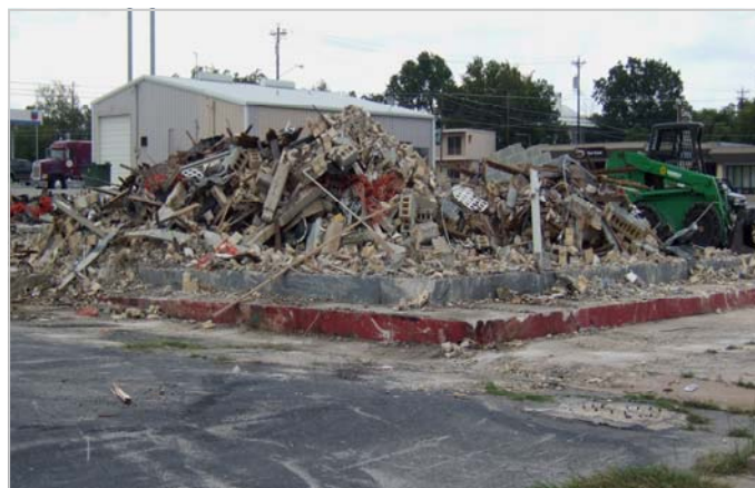
Demolition work begins for the new Walgreens store to be located on the north west corner of the intersection of Highway 29 and 281 in Burnet.
