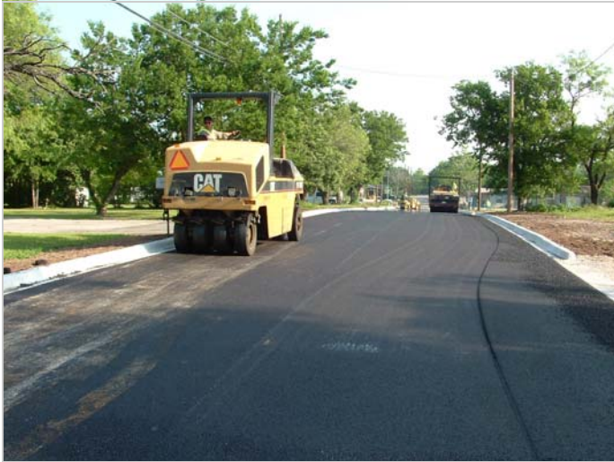
O'Neil Street in southeast Burnet receives new curb and gutters and pavement during the street improvement project.
